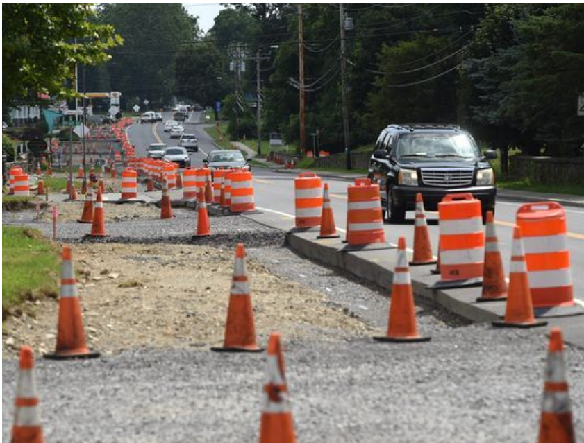
A view of the construction happening along Route 9 in Hyde Park. (Photo: Alex H. Wagner/Poughkeepsie Journal)
