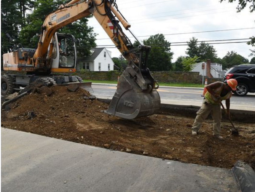
A view of the construction happening along Route 9 in Hyde Park. (Photo: Alex H. Wagner/Poughkeepsie Journal)
