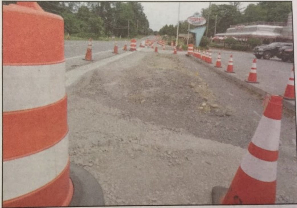
A portion of the east side of Route 9 in Hyde Park is under construction to improve pedestrian and bicycle access and to install landscaping to beautify the area. Photo by Curtis Schmidt
